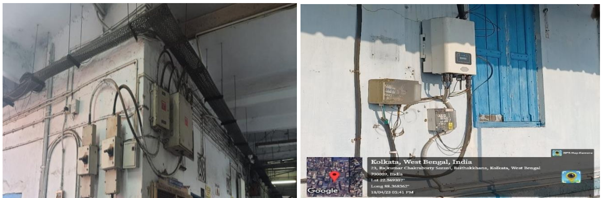
Figure 1. Power house and energy distribution module of Bangabasi Evening College
