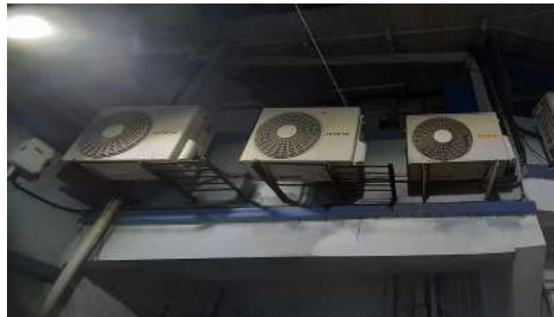
Figure 5. A.C. installed at Bangabasi Evening College
