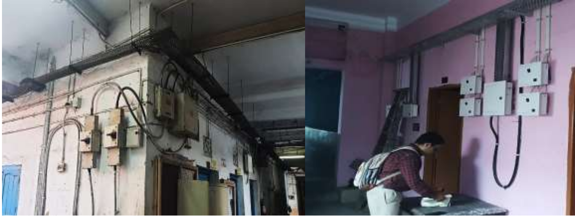
Figure 1. Power house and energy distribution module of Bangabasi Evening College
